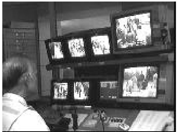
Figure 3: The technology in the Station Ops room
